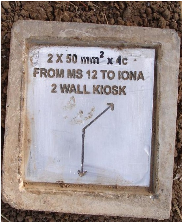
Change or Direction Cable Route Marker
